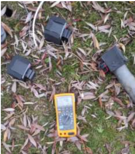
Figure 4.5.2 Holes were made in the lawn for aluminum rods of different lengths, into which the rods were inserted. The bottom 100 mm of the aluminum rod was without pipe insulation.
