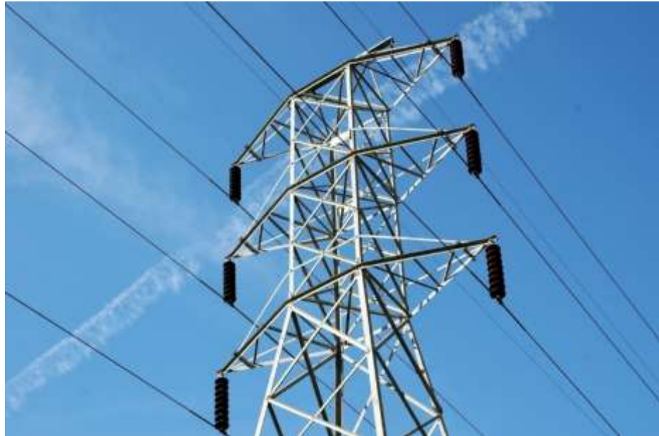
Figure 2.1 High voltage power line.
